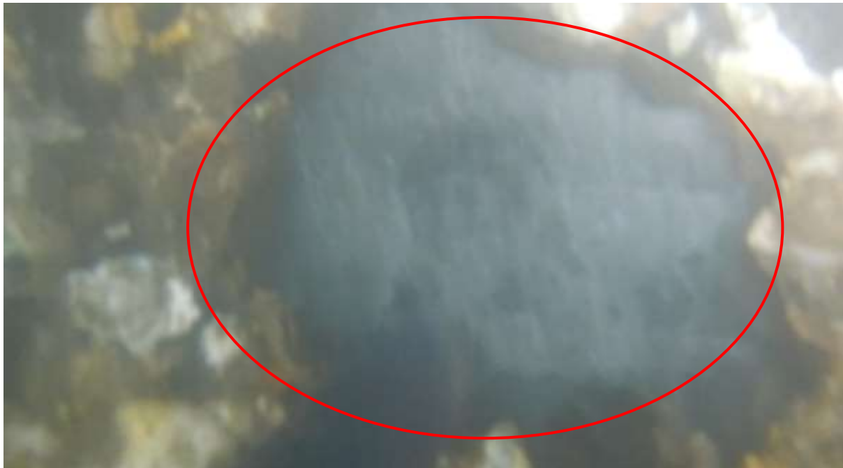
Fig 3.8: A view of distress in a pile-2
