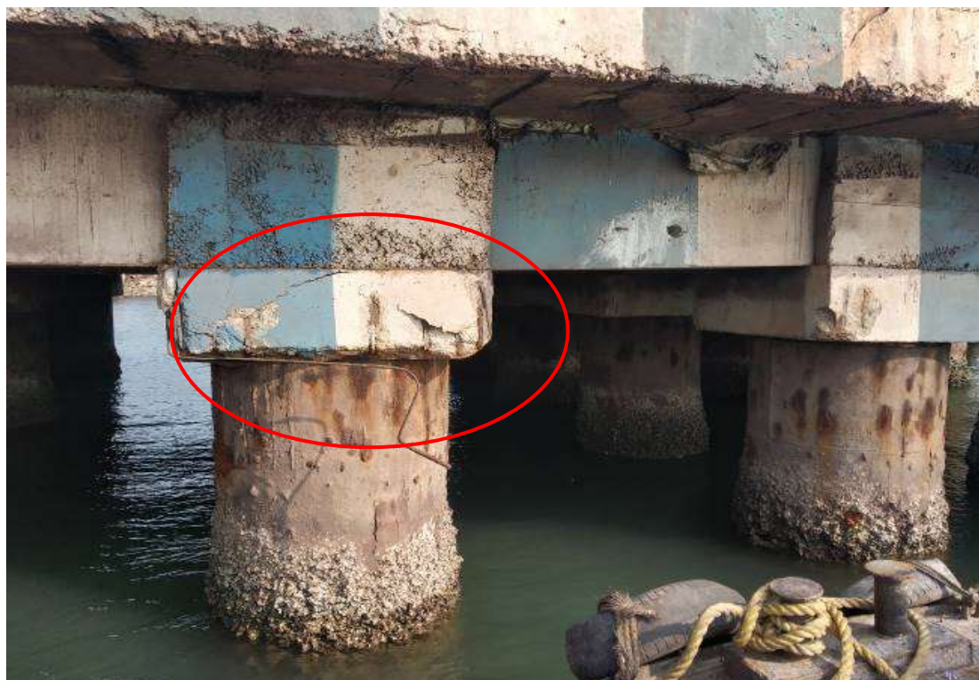
Fig 3.7: A view of the cracking/spalling of concrete and exposure of rebar noticed in RC Pile cap in the berthing side
