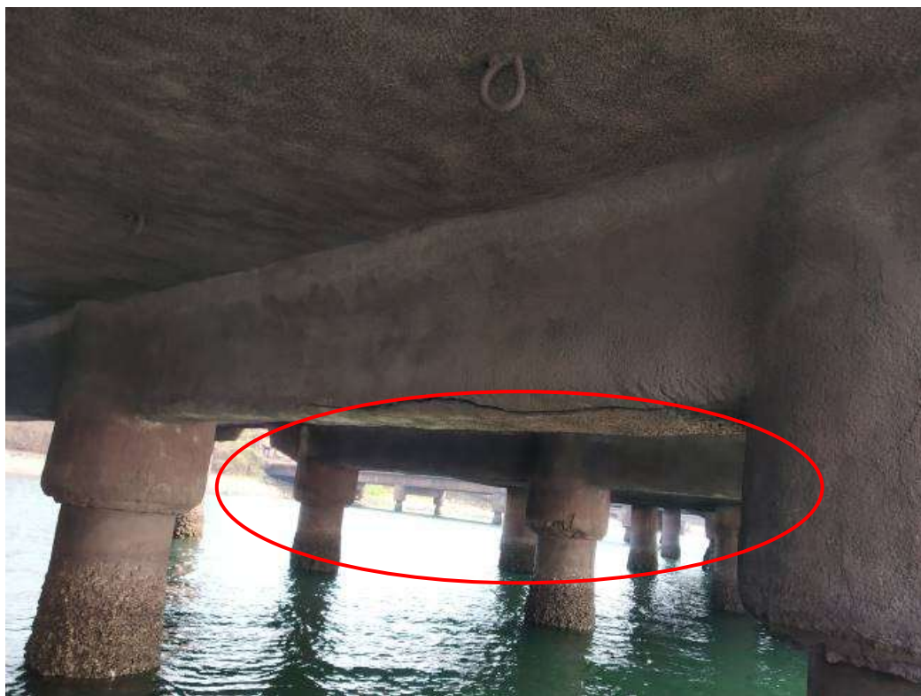
Fig 3.3: A view of the cracking noticed in the RC Beam between the Piles
