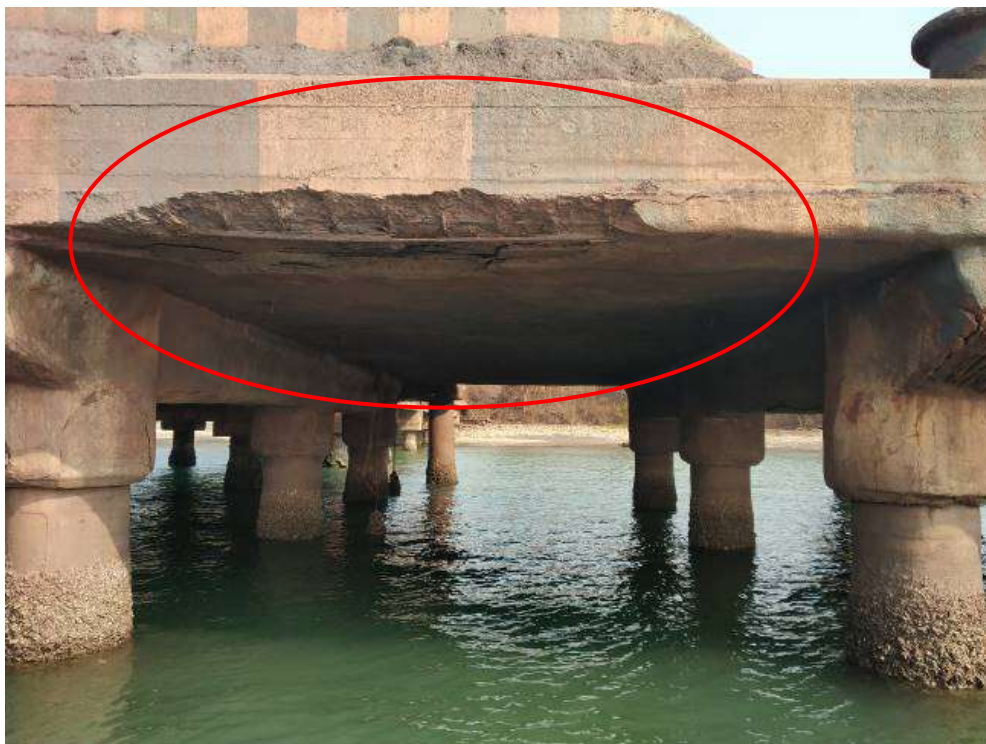
Fig 3.5: A view of the spalling of concrete and exposure of rebar noticed in RC Deck slab on the berthing side
