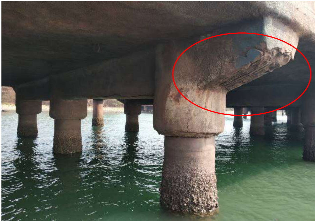
Fig 3.6: A view of the spalling of concrete and exposure of rebar noticed in RC cantilever beam on the berthing side
