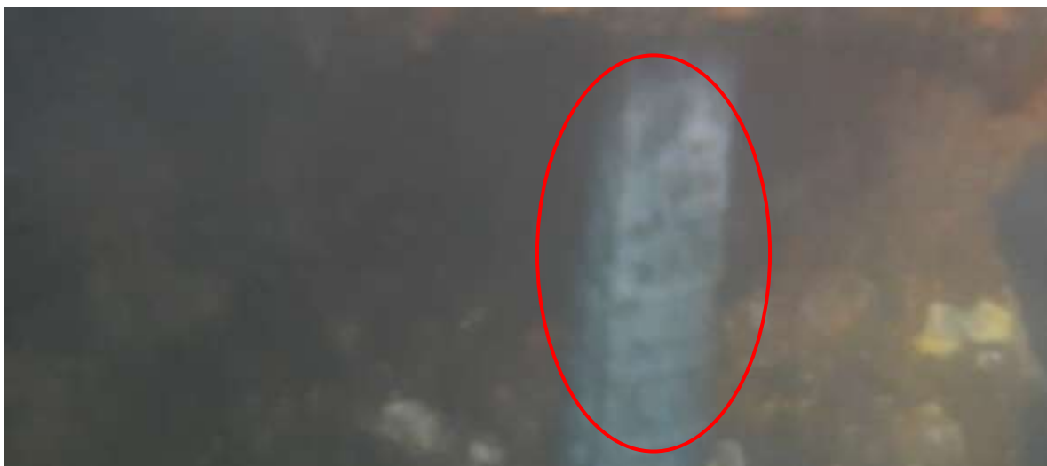
Fig 3.10: A view of exposure of reinforcement in a pile
