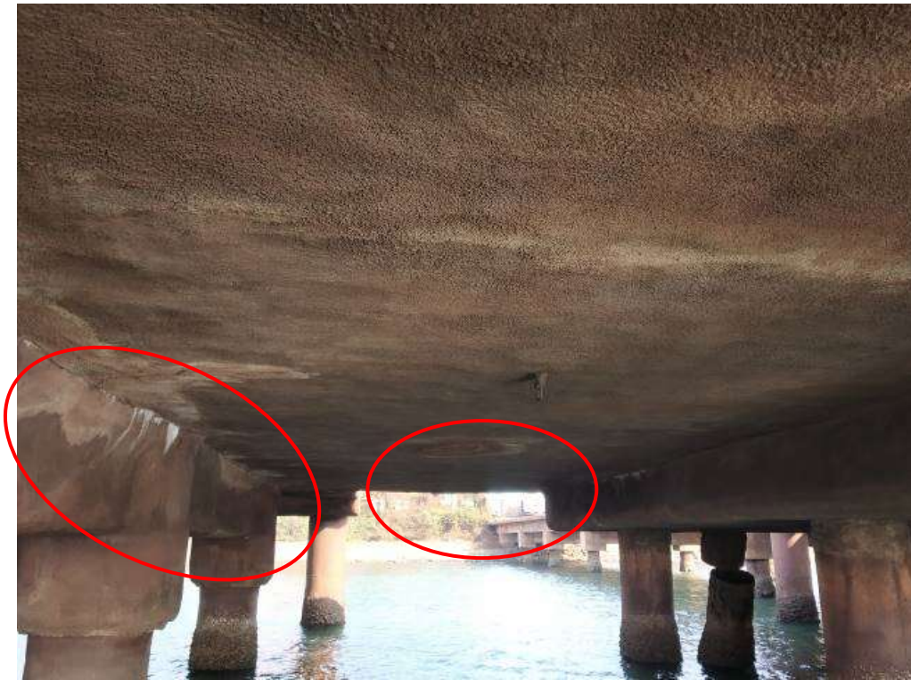
Fig 3.4: A view of the leaching noticed in the bottom of the RC deck slab
