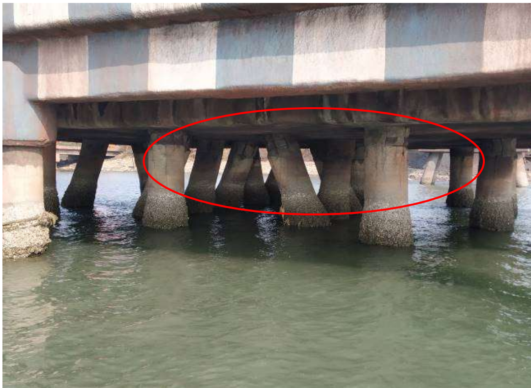
Fig 3.1: A view of the spalling of concrete and exposure of rebar noticed in the Piles
