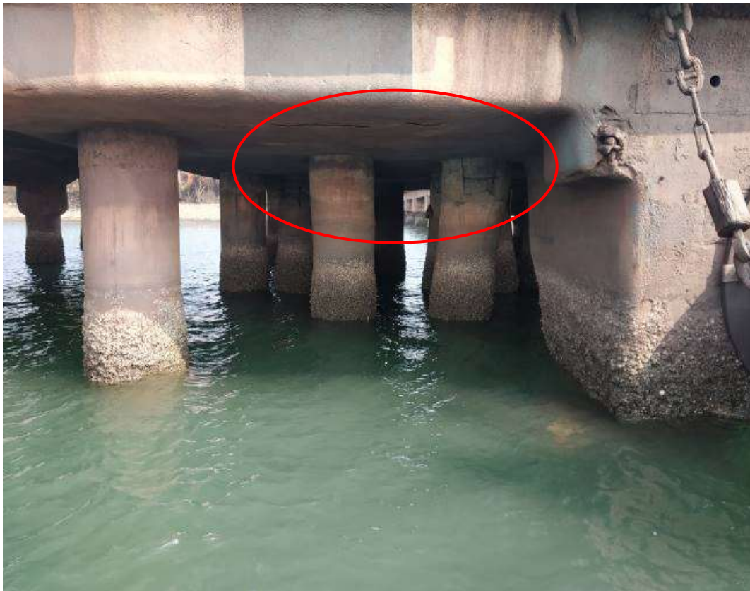
Fig 3.2: A view of the cracks noticed in the bottom of the RC group pile cap
