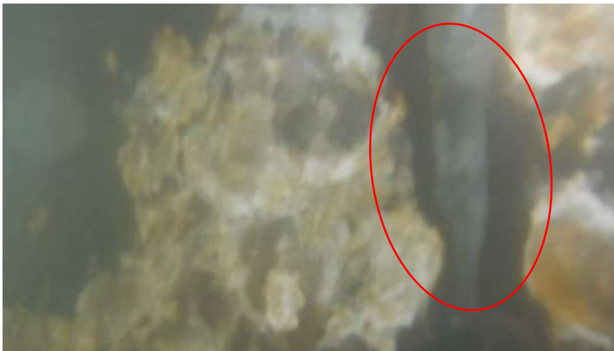
Fig 3.11: A view of exposure of reinforcement in a pile-2
